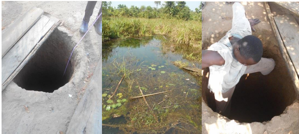
Gibina Village well, drilling began on January 2, 2017. Well is currently 12 meters deep, and will be complete by March 15, 2017. Center: current water source, contaminated for human consumption as an ecosystem exists within it. The water stream will dry late February and will not collect water again until July. Right: Mr. Sam & Co. worker going down to dig the hole further.
