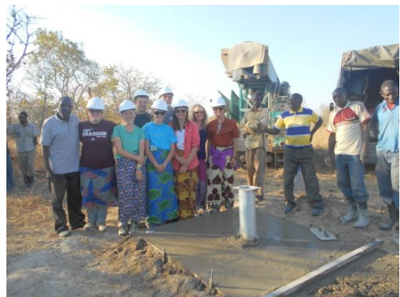
Engineers Without Borders (EWB)-Mississippi State University drills its first well in Siamabwe Community, Simwatachela, Zambia: August 2014.
