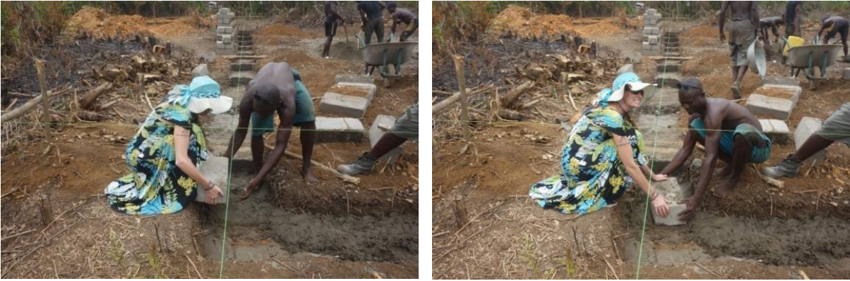
Laying the first block on the foundation of our house is a tradition here in Sierra Leone.
